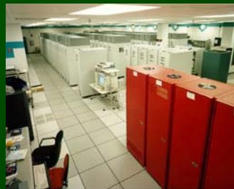
Intel ASCI Red .850 Megawatts
