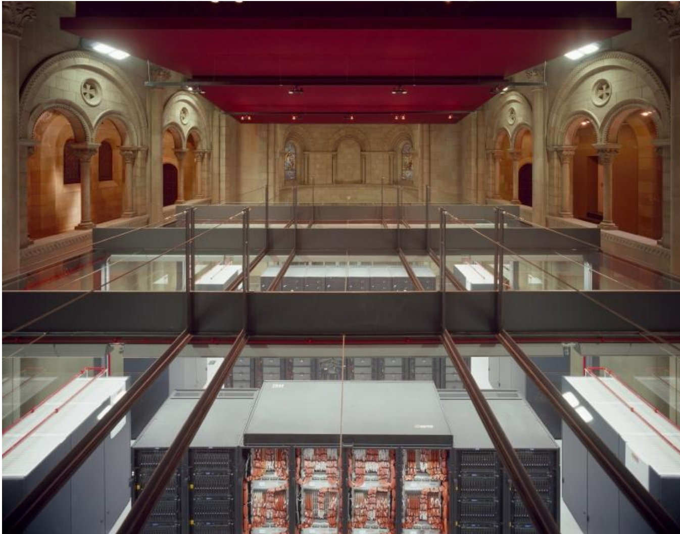
MareNostrum Cluster in Barcelona. The central Myrinet-2000 switch has 2560 host ports. Photo courtesy of IBM.
