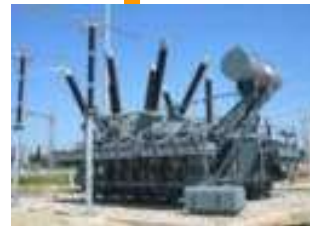
Phase Shifting Transformers
