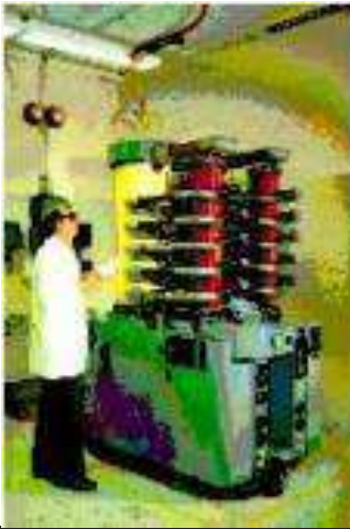
Mercury Arc Valve HVDC (Phased out)
