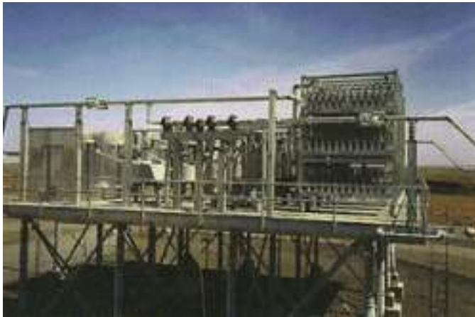
1 st Thyristor-Controlled Series Compensation (TCSC) Project
