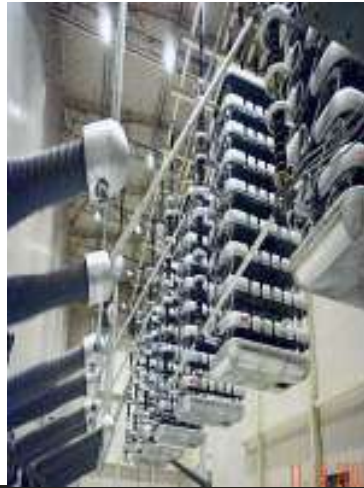
Thyristor Valve HVDC Classic
