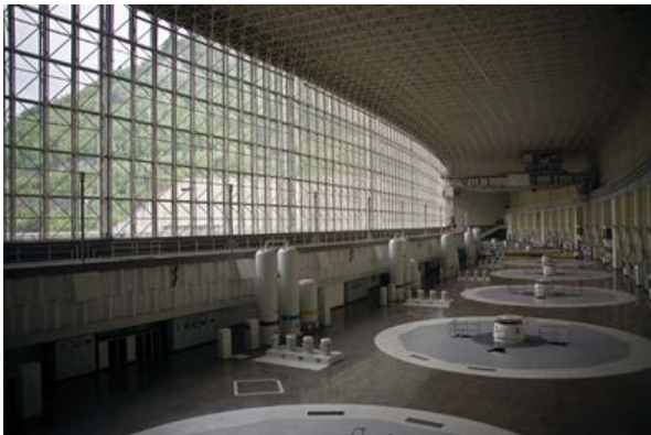
Before the accident
