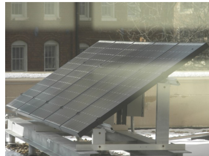
(a) Solar panels
