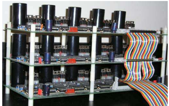
Fig. 8. 10 kW multilevel inverter prototype.
