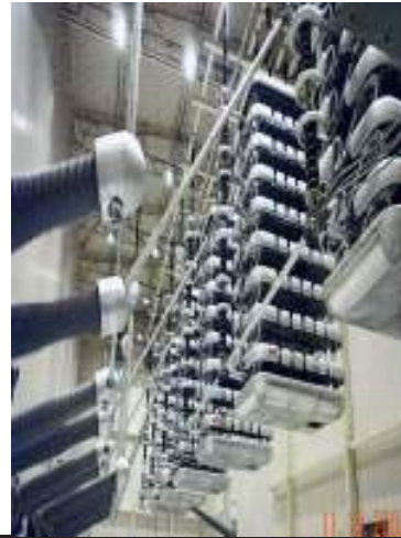
Thyristor Valve HVDC Classic
