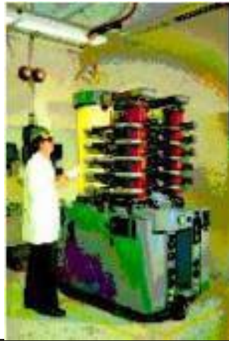
Mercury Arc Valve HVDC (Phased out)
