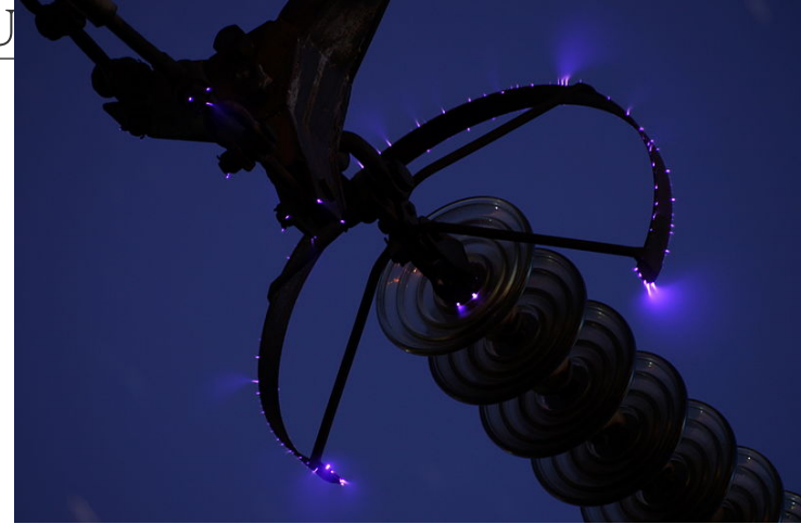
Corona discharge on insulator string of a 500 kV line (source: wikipedia.org)
